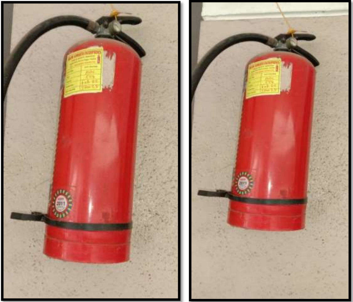
Photo No. 8 Fire Extinguisher
